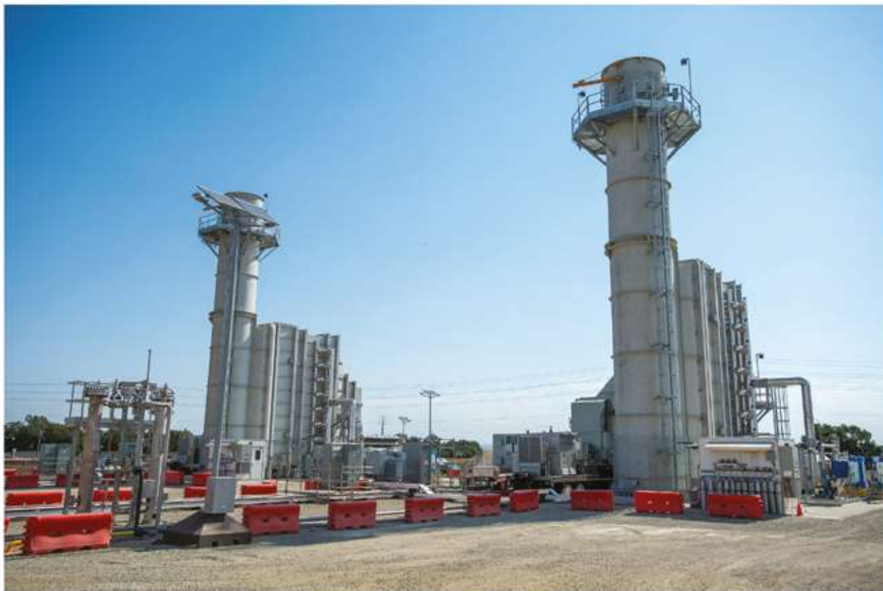
GE's gas turbine fleets already play an important role in Vietnam's energy transition
